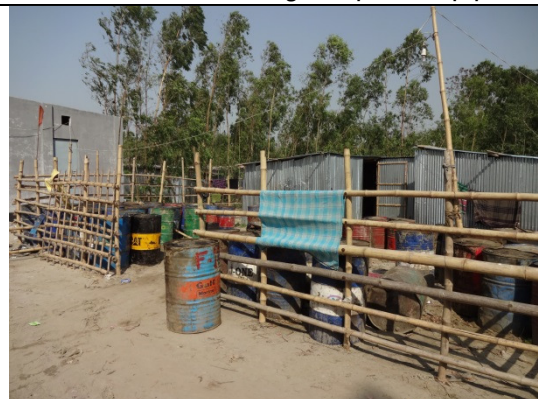
8. Fencing of fuel & lubricant storage
