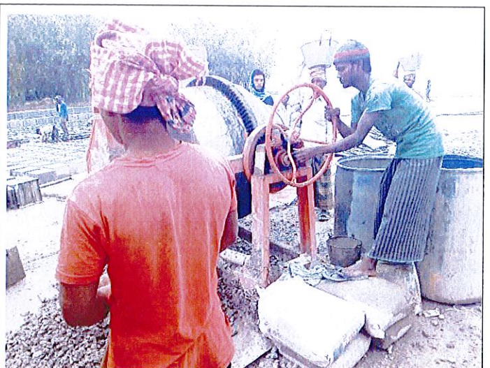
2. Concrete mixture machine is driven without safety equipment
