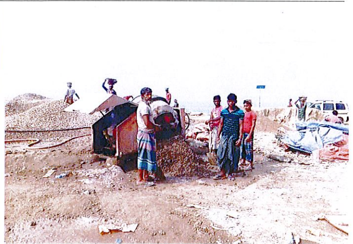
2. Concrete mixture machine is operating without safety instrument.
