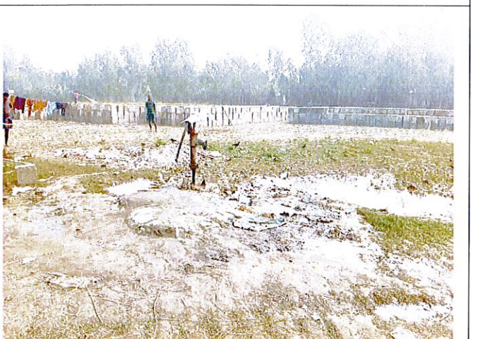
6. Tube well with no protection directly discharging in nature
