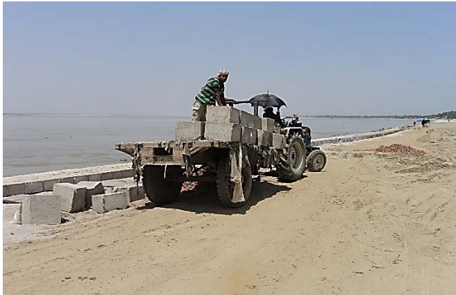
1. Vehicle is carrying C.C. block for placing on slope of protection work
