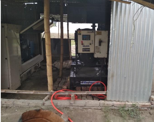
1. Protected generator room
