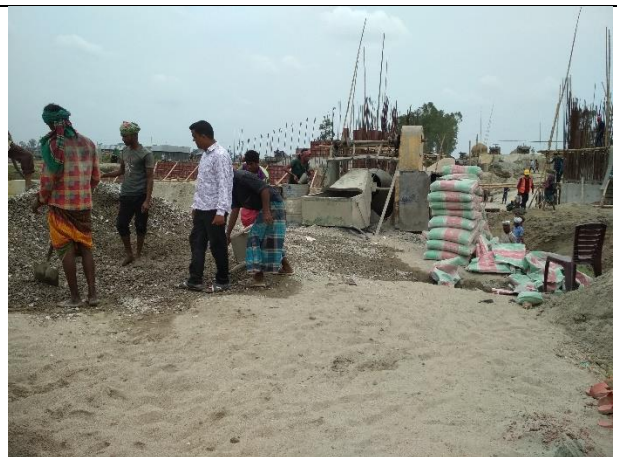
4. Labours are working without wearing PPE
