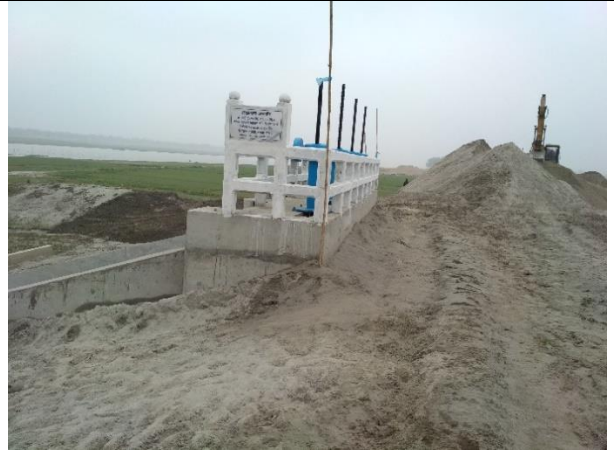
2. Completed 4 vent Regulator
