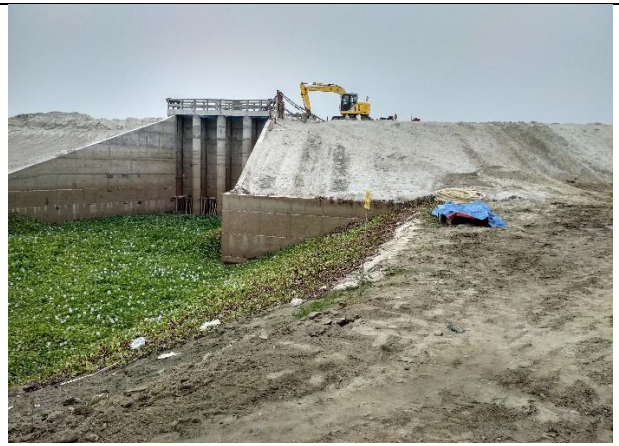
4. Completed 4 vent Regulator at Andermanik
