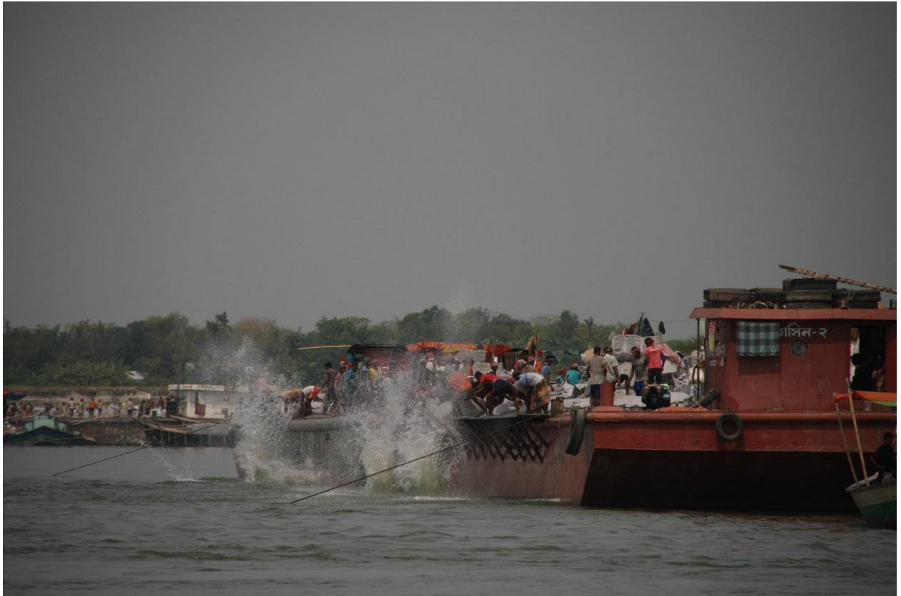
Two dumping sets in action covering a 65m wide strip each, 14 March 2016
