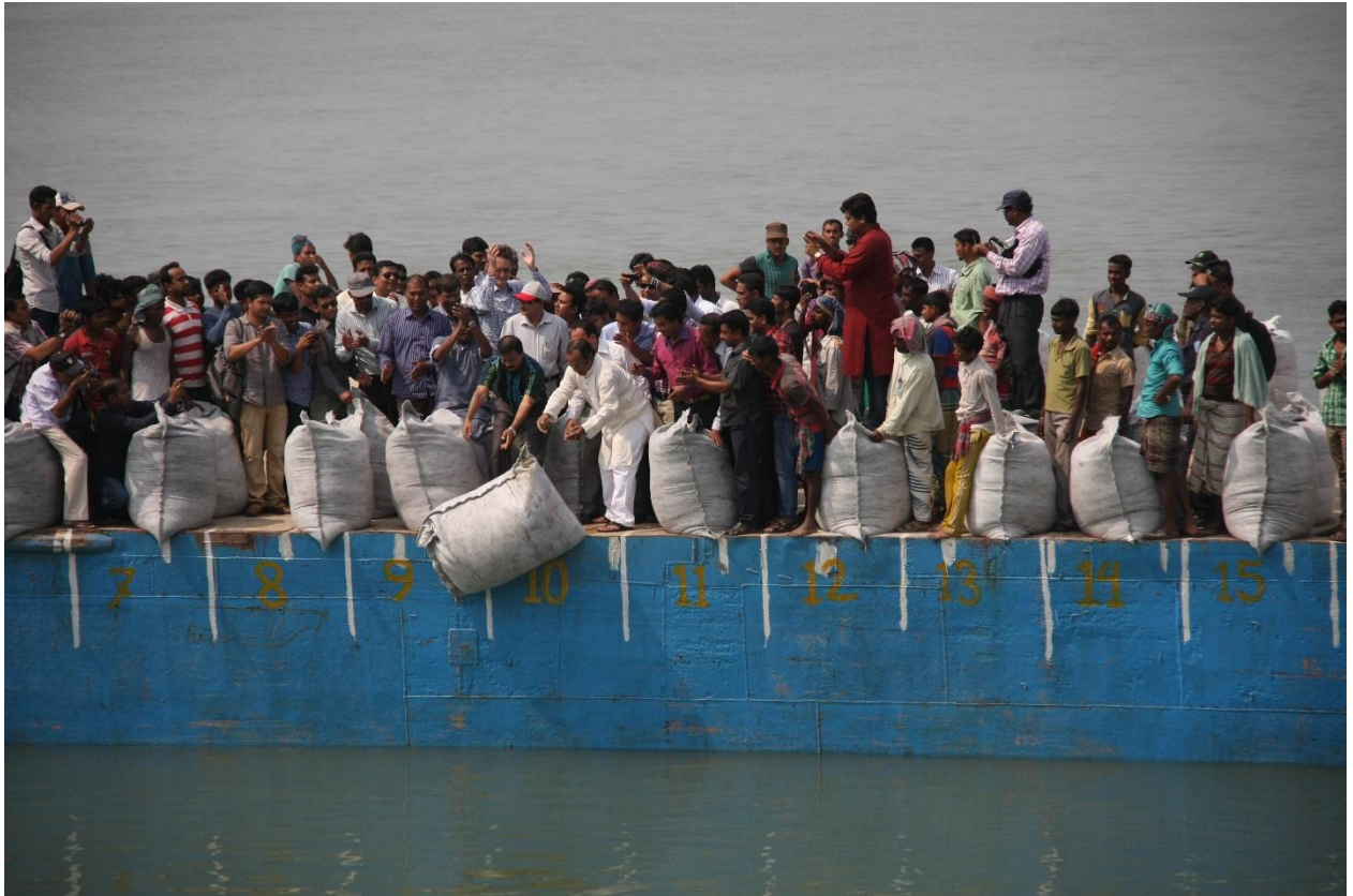
Inauguration of work at Zaffarganj – the honorable MP A M Naimur Rahman (Durjoy) and the Project Director Aminul Haque dump the first bag of the underwater protection on 8 March 2016
