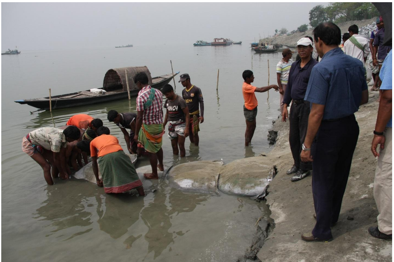
Inauguration of wave protection work at Harirampur in presence of the head of the Task Force and the Project Director on 12 March 2016
