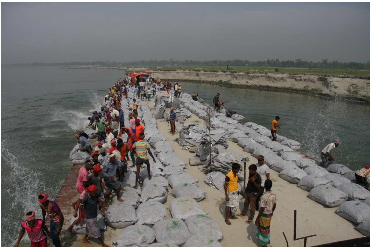
Commencement of dumping of geobags in Harirampur from both sides of the barge on 12 March 2016
