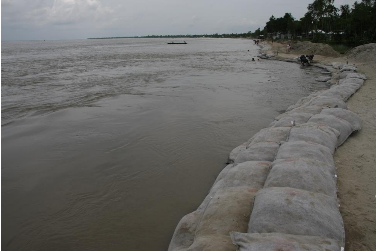
Repair of temporary wave protection in area of angular flow attack, Chauhali, 24 June 2016
