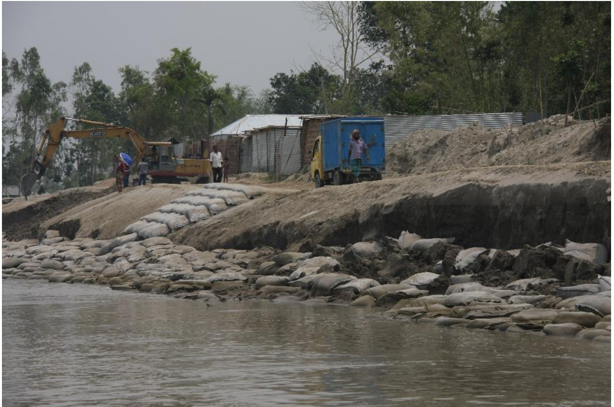
Wave damage under repair at Chauhali on 10 May 2016
