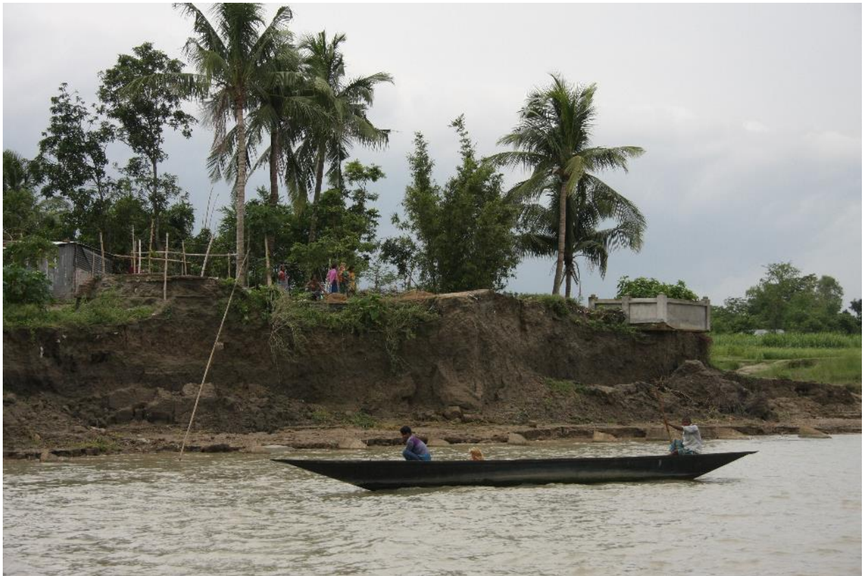
Erosion upstream of Zaffarganj protection on 24 June 2016
