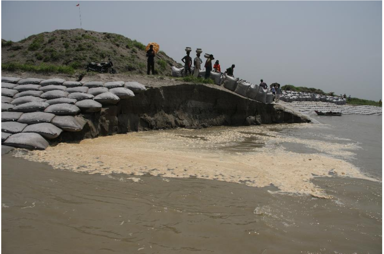
Small erosion of temporary wave protection at Harirampur on 26 May 2016
