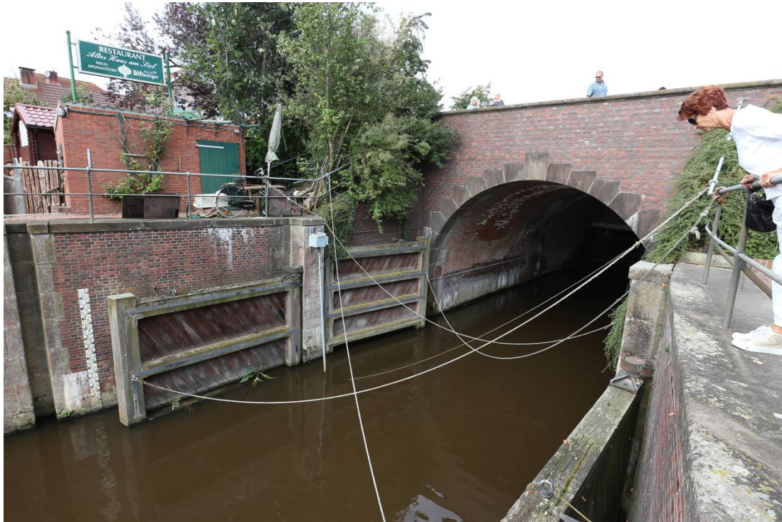
Figure 4. Sluice gate with road bridge for draining a canal into the tidal river Ems
