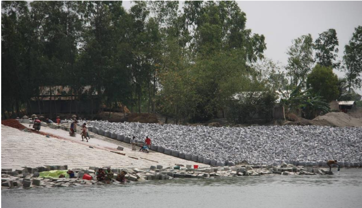
Chauhali construction of permanent wave protection with alternative key and repair of geotechnical failure zone.
