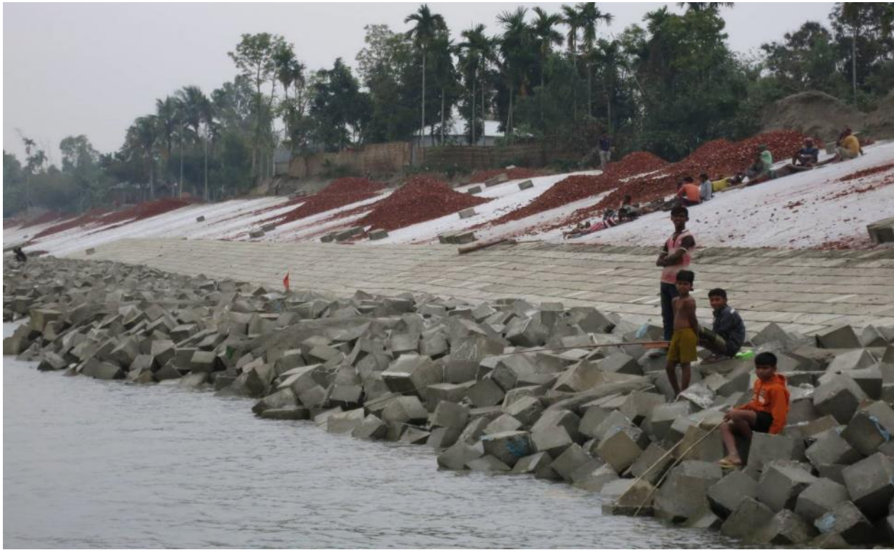
Chauhali low water key (blocking access to the river) and construction of permanent wave protection
