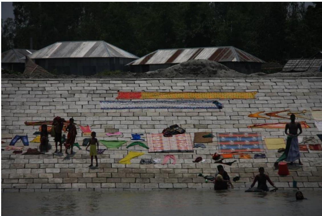
Chauhali: the completed revetment allows the local population easy access tot he river
