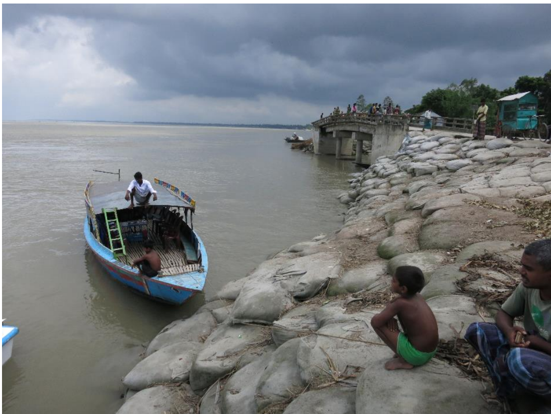
Photo 2. Temporarily protection at bridge after slope failure at Chauhali, 1 Oct 2017
