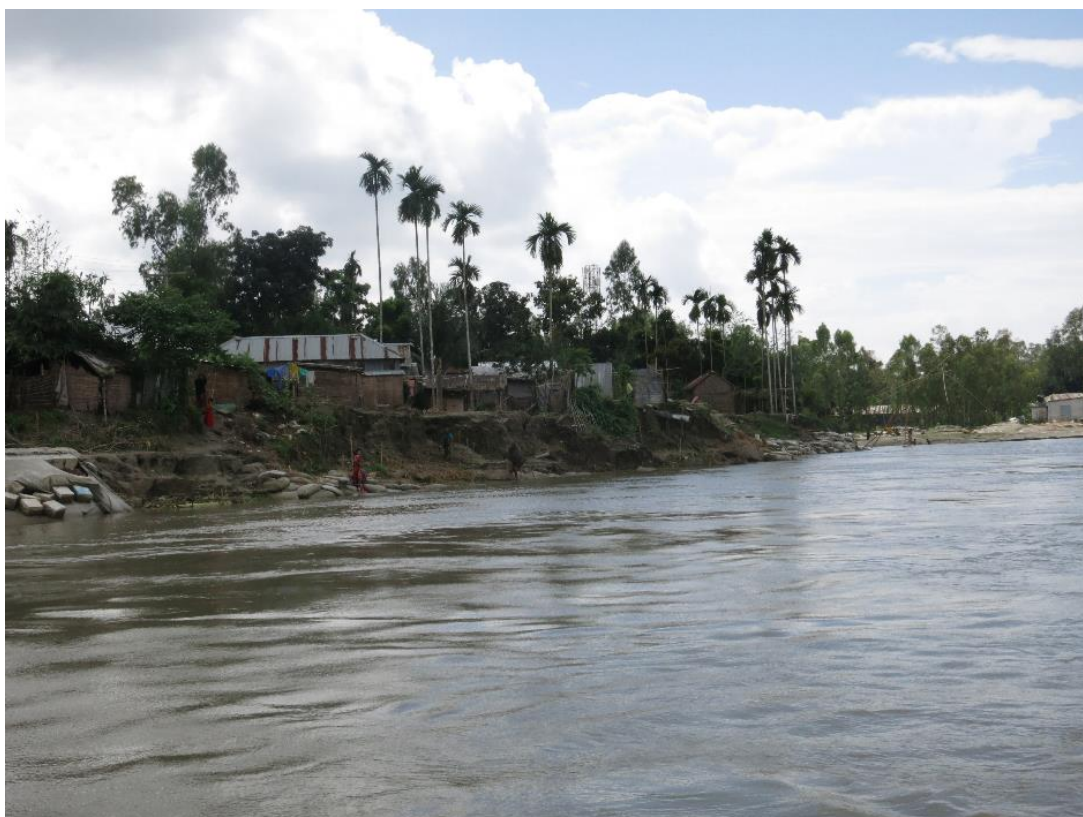
Photo 4. Chauhali local failure of upper slope with temporary repair works, 1 Oct 2017
