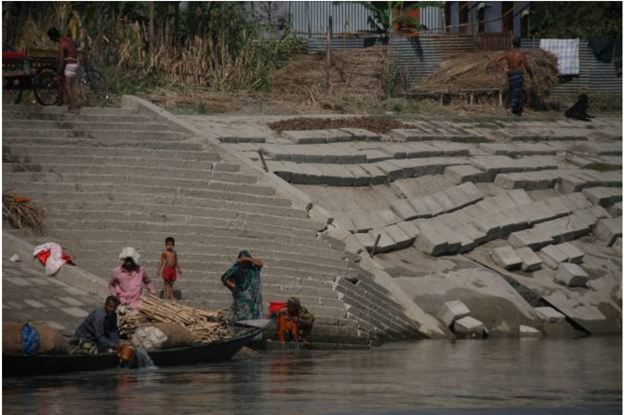
Photo 7. Localized revetment damage at Kojjuri, 1 December 2017
