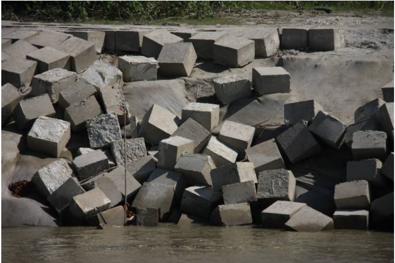
Photo 3. Surficial slope failure at Chauhali, with concrete blocks to be salvaged, 24 November 2017
