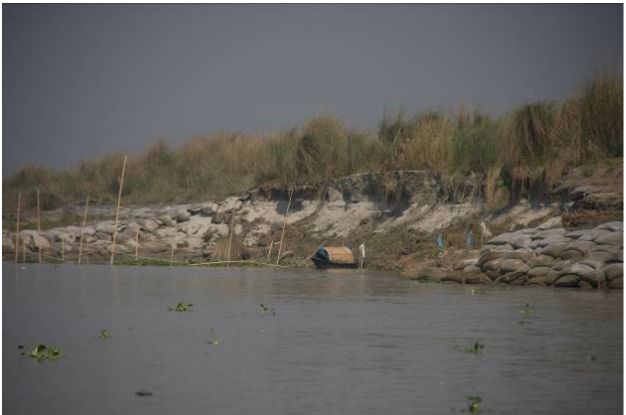
Photo 12. Localized damage of temporary wave protection at Harirampur, 12 December 2017
