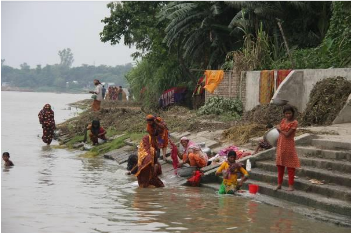
Riverbank Protection at the PIRDP, built between 2004 and 2008 – in good condition after 10 years
