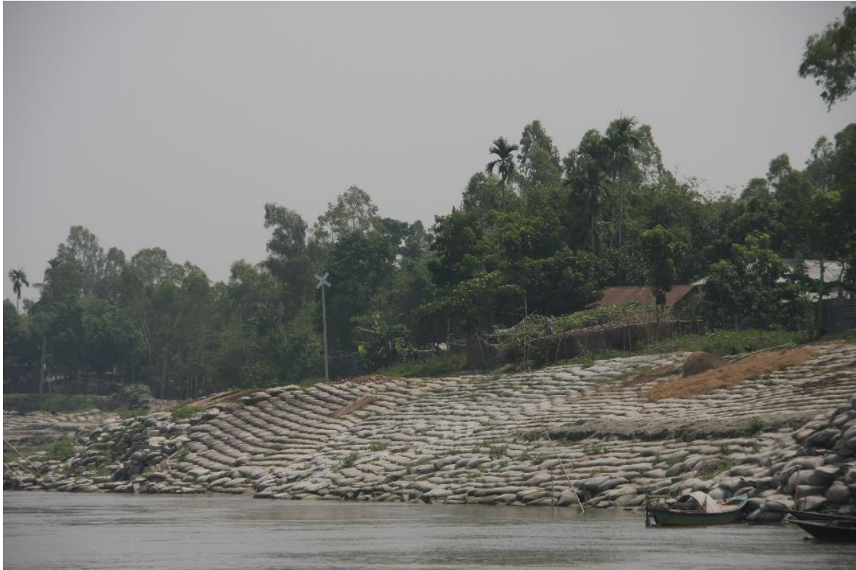
Figure K3: Chauhali, stabilized bank requiring future flattening and berm widening, 20 April 2019
