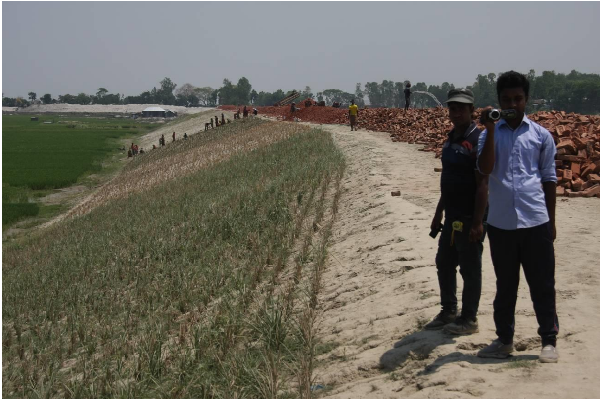
Figure K7 : Harirampur embankment, plantation of vetiver on countryside slope, contract package 4, 20 April 2019
