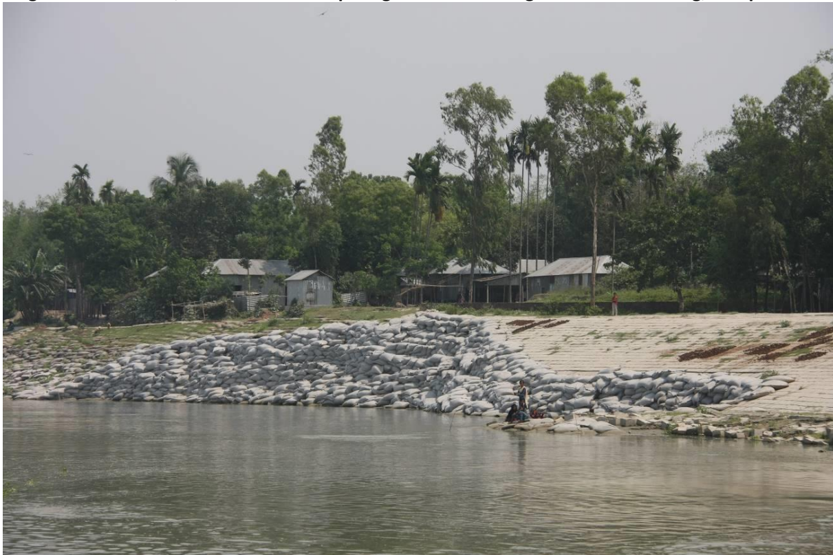
Figure K4 : Chauhali, stabilized latest slope failure at km ... (Feb 2019), 20 April 2019
