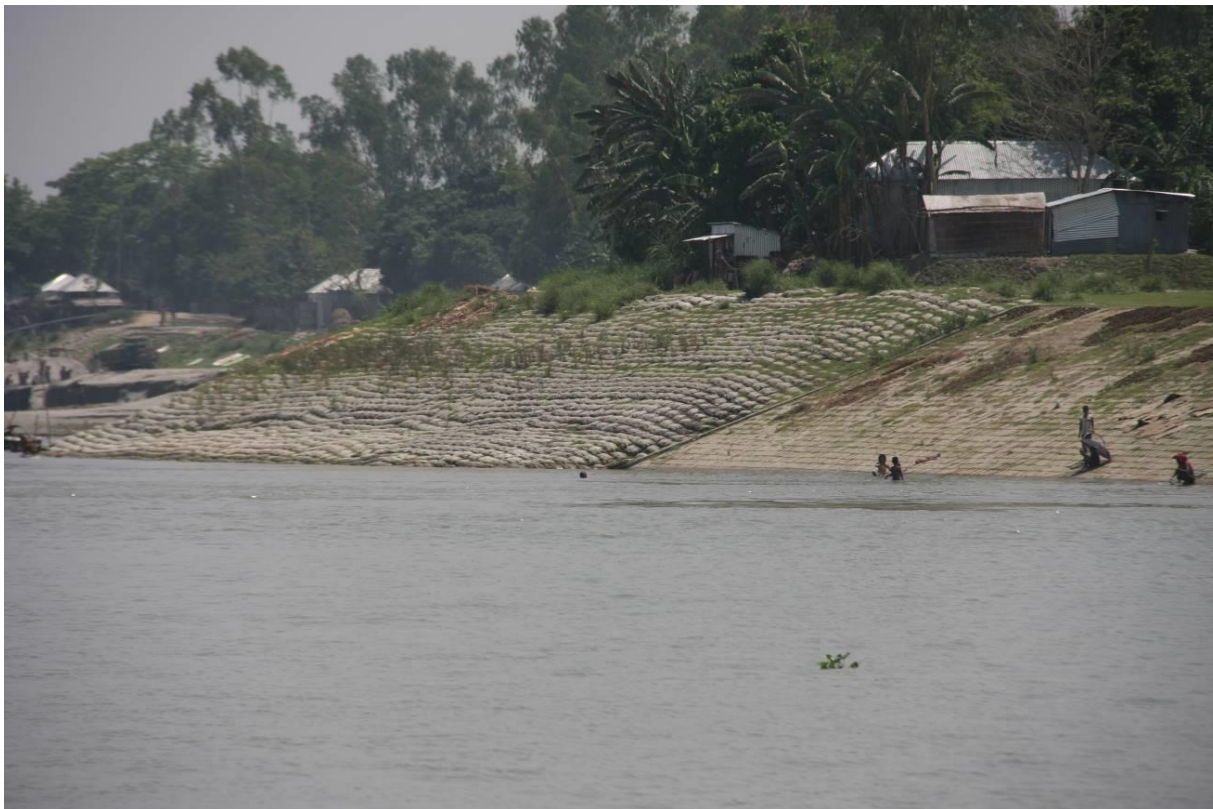
Figure K 10 :PIRDP, the grout-filled mattress installed in 2006 has performed without maintenance
