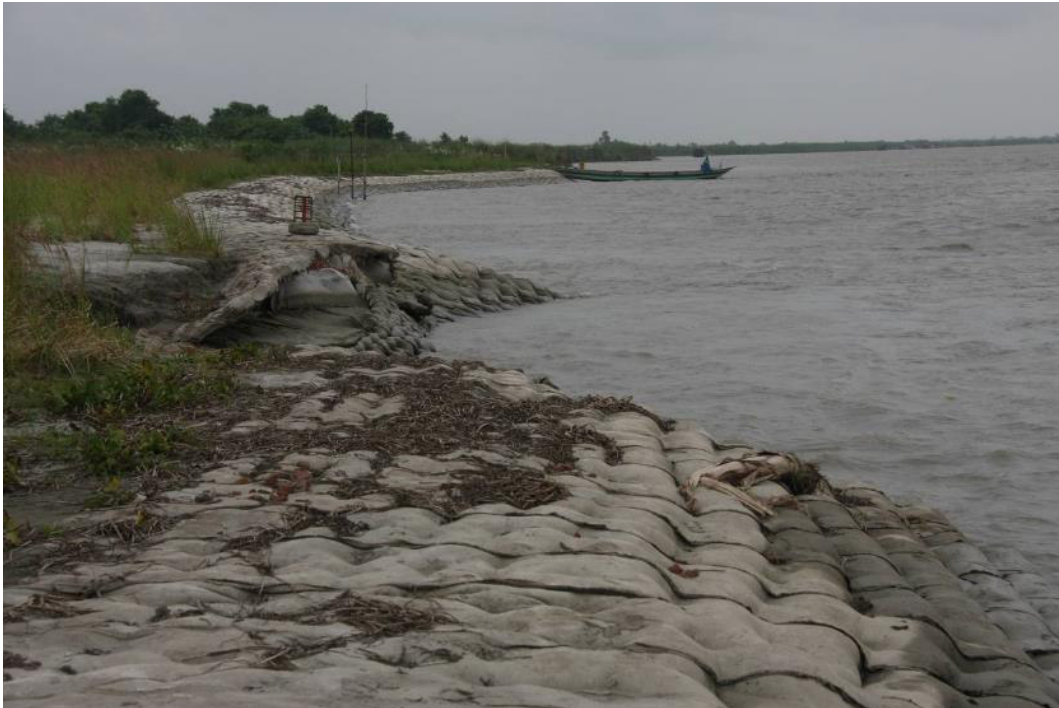
Figure L-13 Harirampur damaged section of grout-filled jute mattress, 13 Sep 2019
