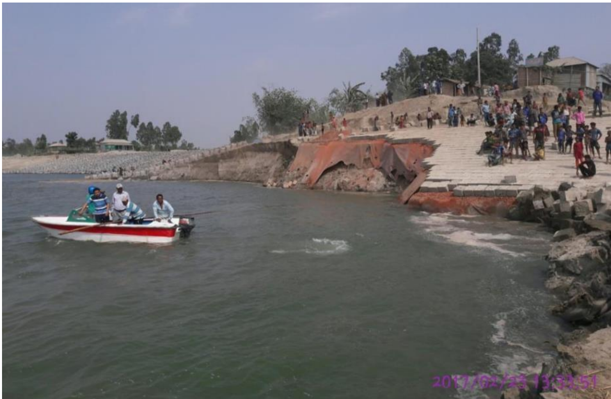
Figure 3-12 Bank failure in Chauhali
